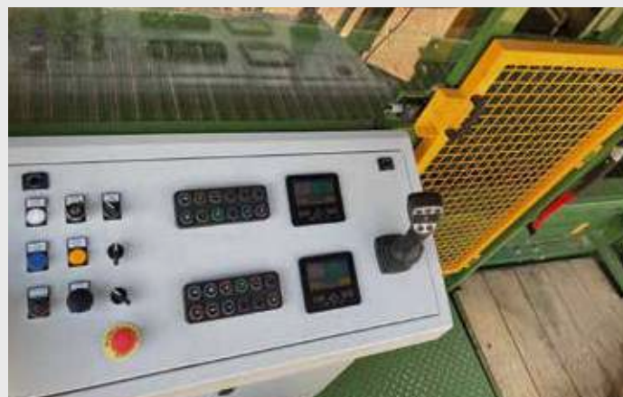
TM-TB - Control panel
